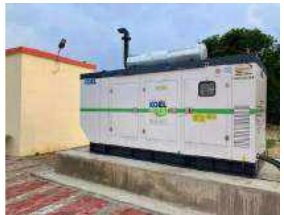
Genset with acoustic Enclosure West Campus
