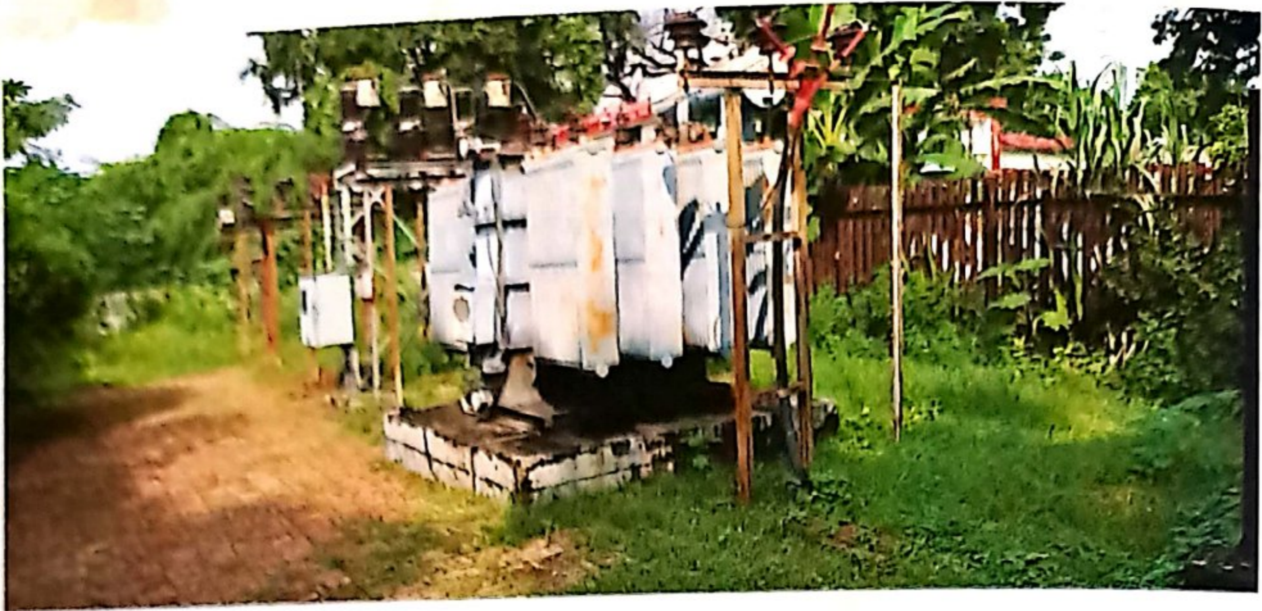
Electrical Sub Station
