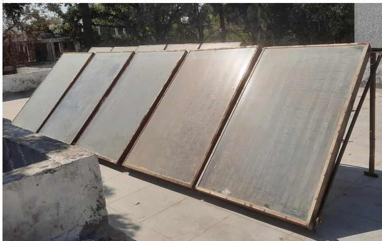
Figure: Solar panels for water heating in hostels
