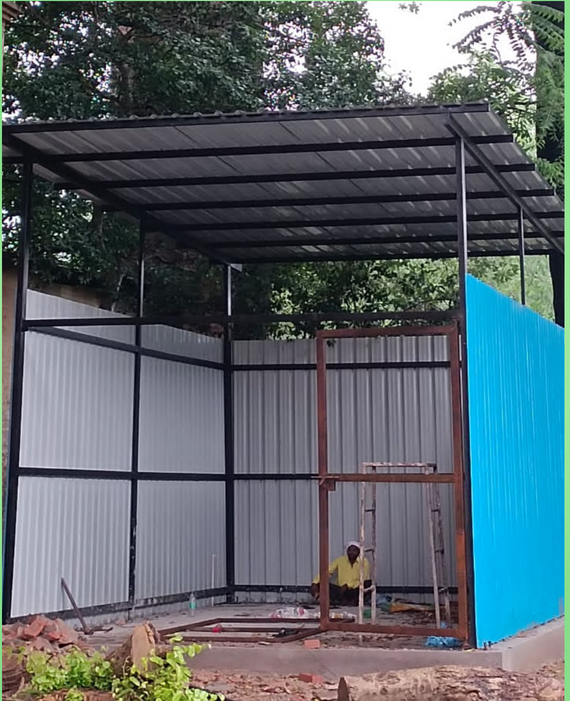
Fig.6 Solid Waste Disposal Facility operated by KNN in the East Campus (Under Construction)
