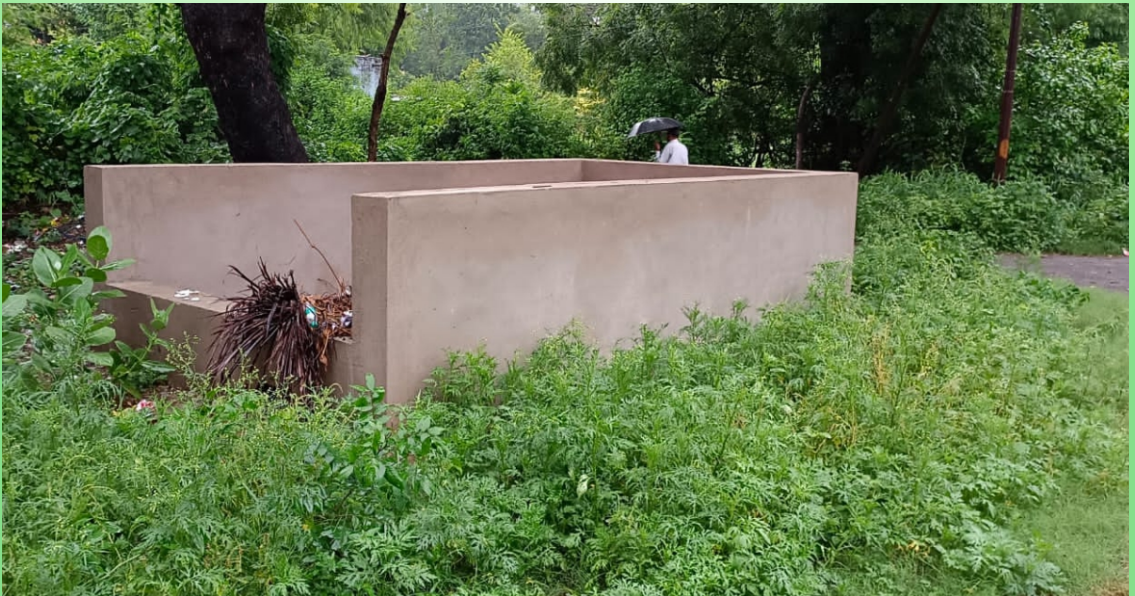
Fig.5 Block Cum Community Storage pit in the East Campus of the University
