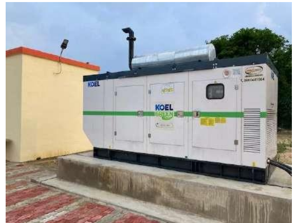
Genset with acoustic Enclosure West Campus
