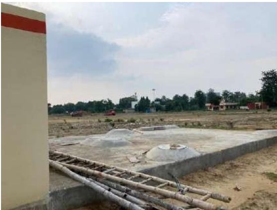
Static Water Tank West Campus
