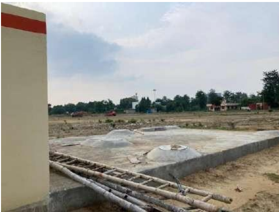
Static Water Tank West Campus
