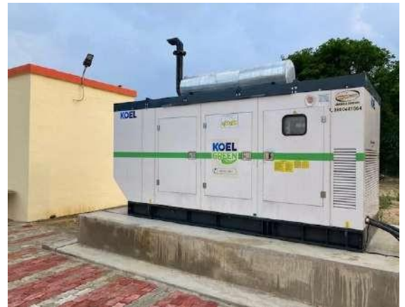
Genset with acoustic Enclosure West Campus
